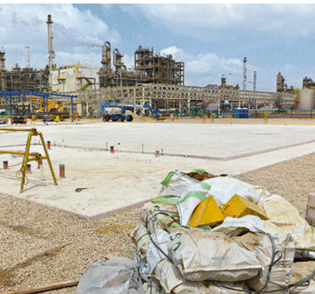
Work is already under way on the expansion of the methionine plant. Plans call for the new components to be integrated into the existing process next winter
