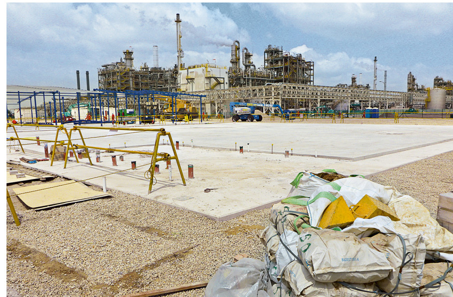
Work is already under way on the expansion of the methionine plant. Plans call for the new components to be integrated into the existing process next winter
